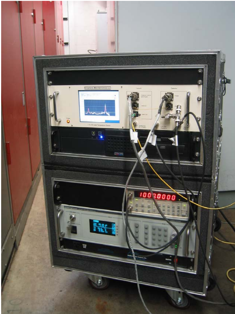
Processing Unit in Power Plant Terminal Room
