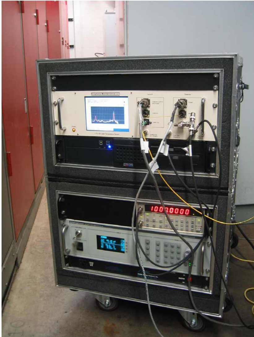
Processing Unit in Terminal Room
