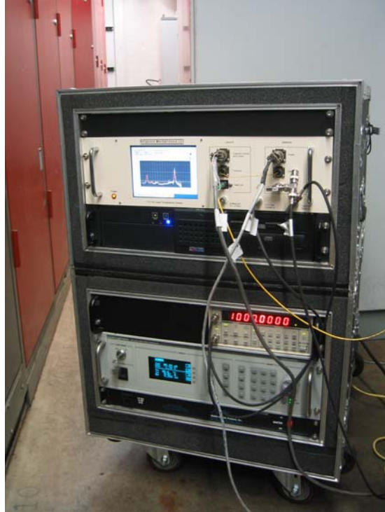
Figure 3. LTS-100 Processing Unit in Power Plant Terminal Room
